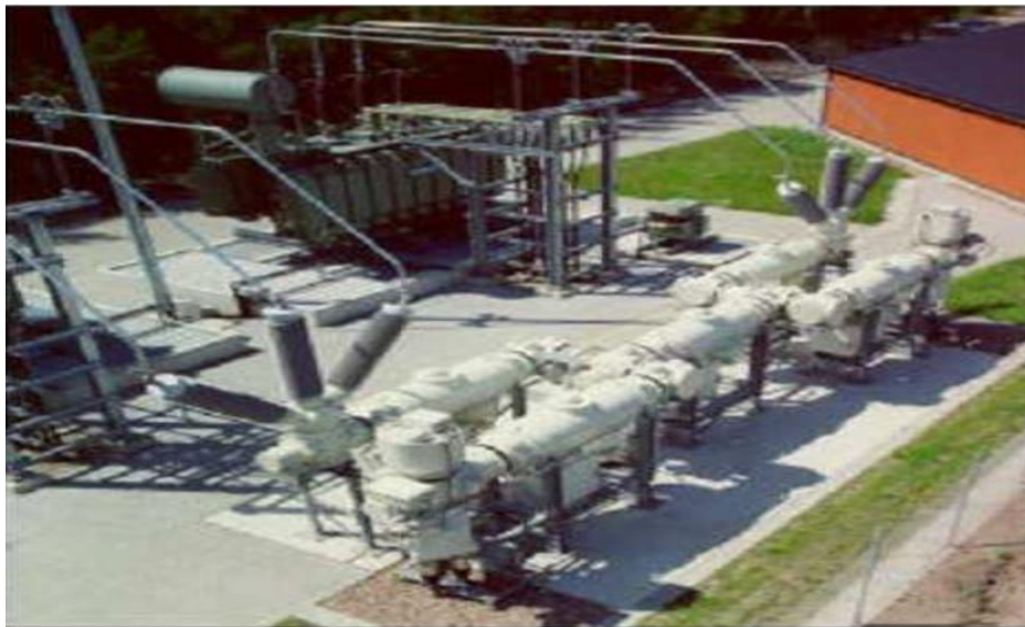
Sl.4.1. HIS postrojenje, 145 kV [9]
