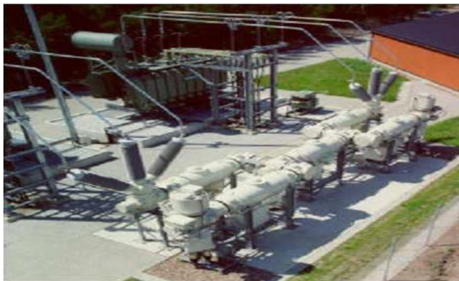
Sl.4.1. HIS postrojenje, 145 kV [9]
