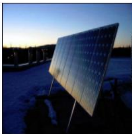
CTS SOLARNI PANELI
