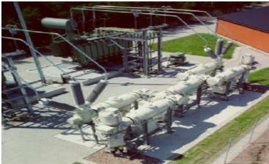
Sl.4.1. HIS postrojenje, 145 kV [9]
